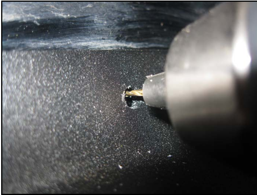
Figure 1. Drilling holes for the upper flange at the top of the hole in the Side Guard.
